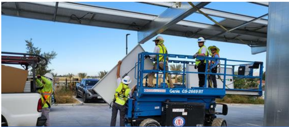
50 kW solar carport
