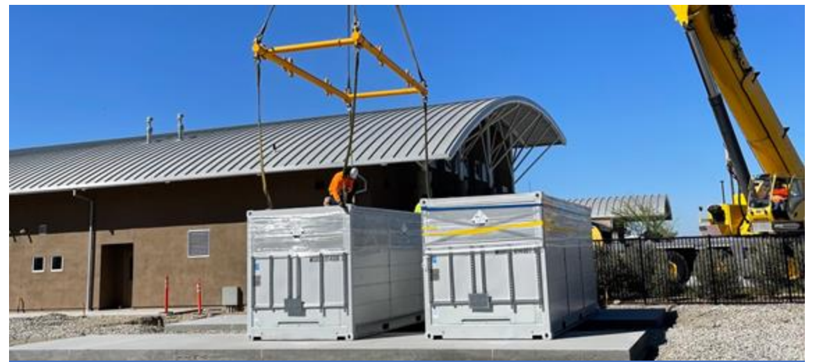
50 kW/500 kWh Vanadium Redox Flow Battery (VRFB)
