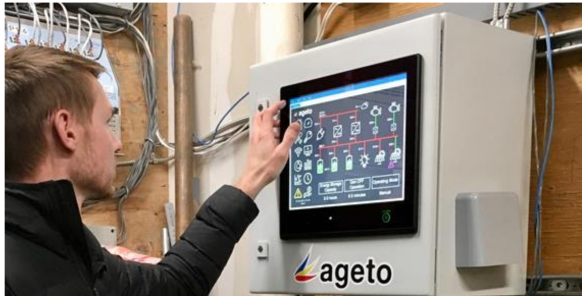
Energy Management System
